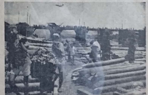
HUNDREDS OF CHINESE COOLIES working under the supervision of the Burma Road Engineers speed repairs on the ancient Yuan Hwo bridge near Chibkiang.
